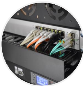
Structured Network Cabling
